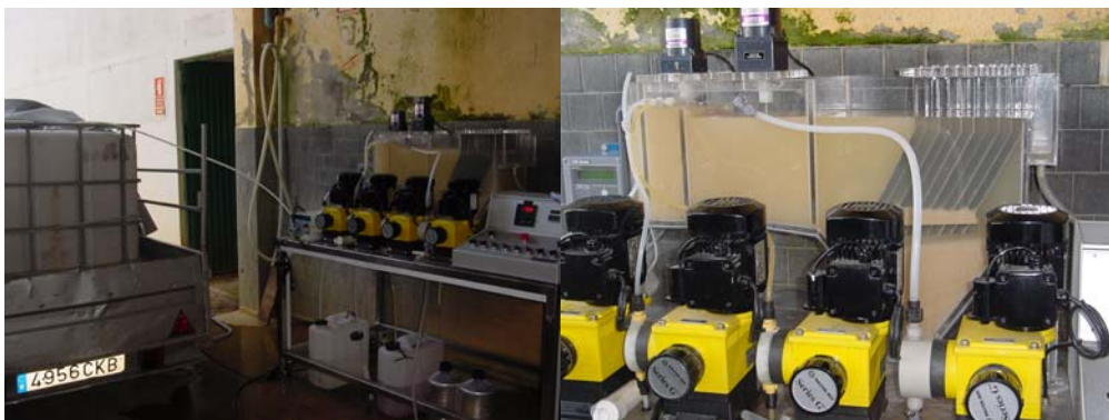
Figure 6-5. In-situ installation of coagulation-flocculation pilot plant.
